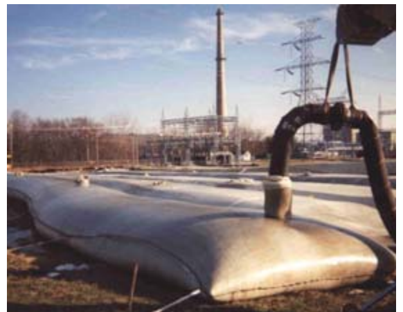
Figure 19. Geotextile tubes can be used to store and dewater hydraulically dredged sediments.
