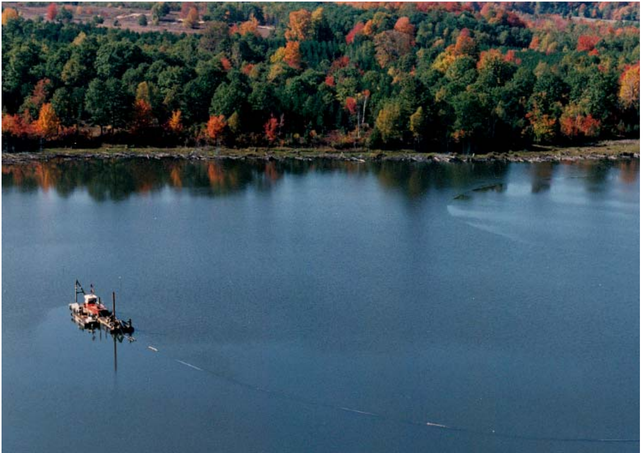
Figure 17. Hydraulic dredging. The floating pipeline is visible behind the barge at the bottom of the photograph.
